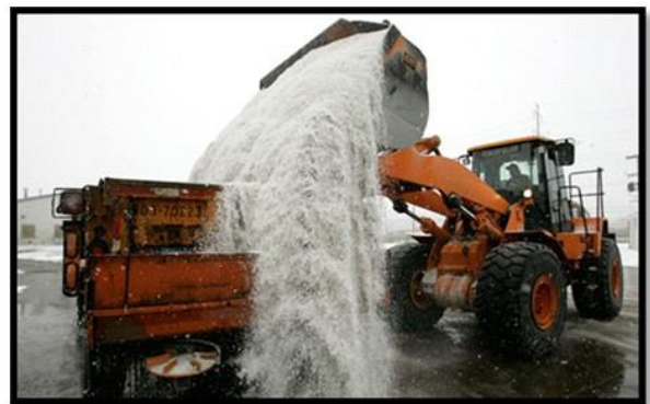
Photo 7. Loading road salt (NaCl) into the back of a plow truck (A.P.)
